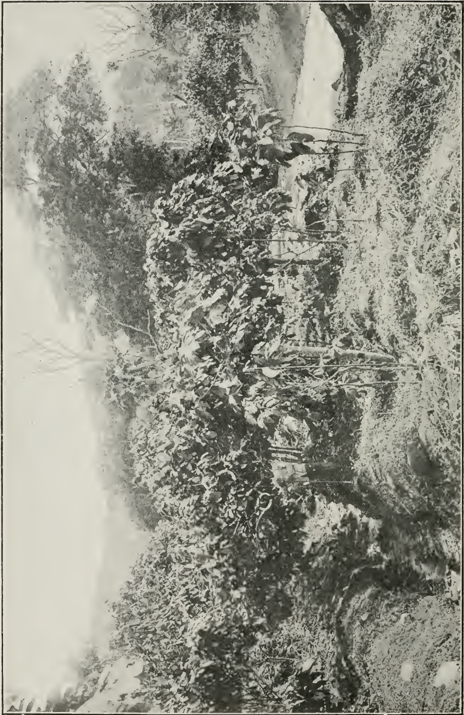
FIG. 54.—DRAINAGE WORKS ON PLANTATIONS ON BANK OF RIO PAPAGAIÓ; ROCA BELLA VISTA.
